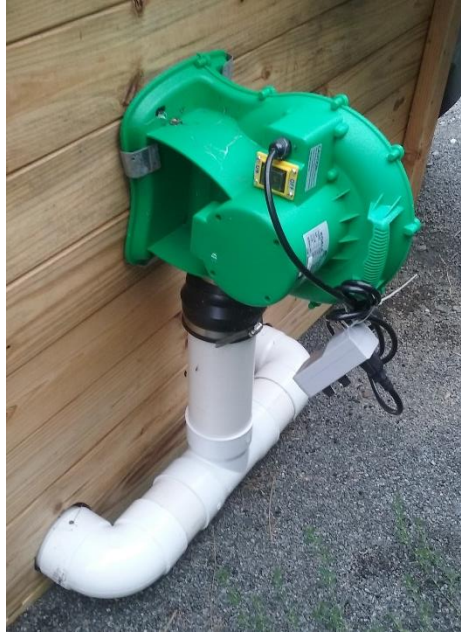
Back side of wooden bin with fan (green) that pumps air into the pile via white PVC pipes at the bottom.
