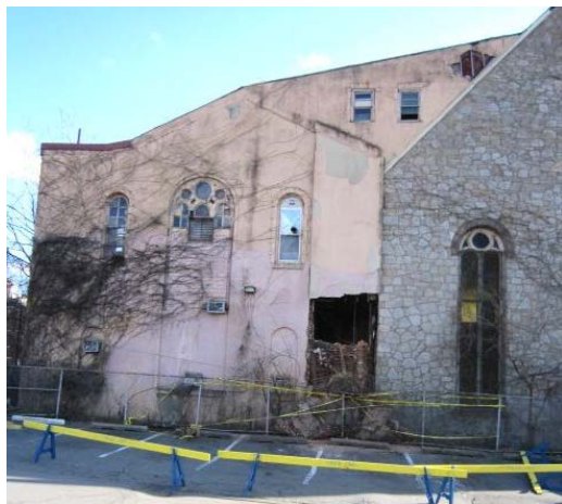
North side of church with annex to left and main church to right. Note rectangular hole in the annex on the lower right side due to partial collapse. Photo April 2018
