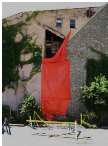
North side of church with another chunk of the annex collapsed. It is partially covered with orange tarp. Photo June 2018
