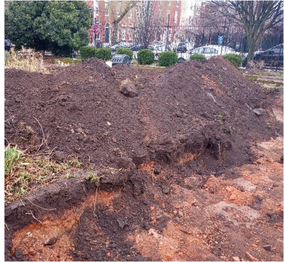
Excavation of part of a plot near the southeast corner. Topsoil was removed and clay substrate is below
